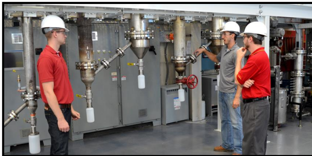
Pilot plant used to design pyrolysis-based 50 tpd MEPS
